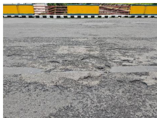
Figure 3. Damage to the Road Pavement
