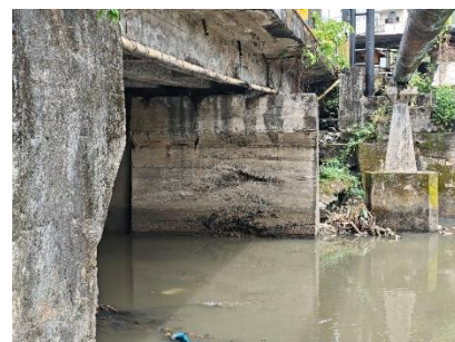
Figure 8. Damage to the Bridge Pier
