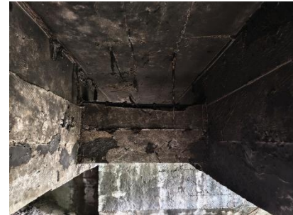
Figure 7. Damage to the Bridge Diafragma
