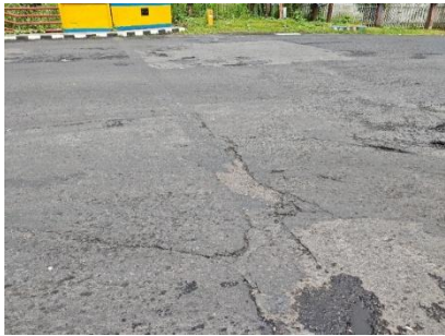
Figure 4 Damage to the Asphalt Expansion Joint
