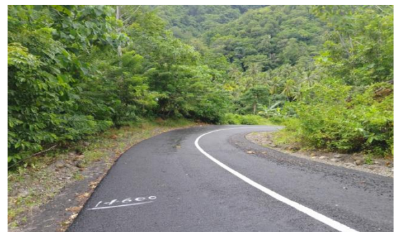
Figure 1. Does not have drainage channels yet
