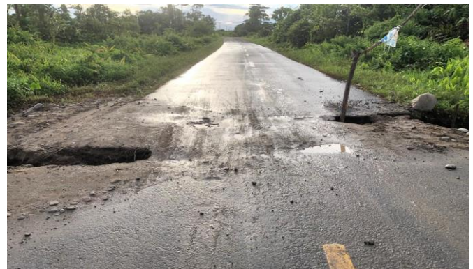
Figure 1. pictures of road damage
