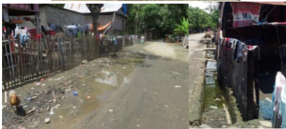
Picture. 5. The drainage system on environmental roads
