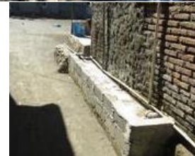
Figure 3. Disposal system in non-stage housing units
