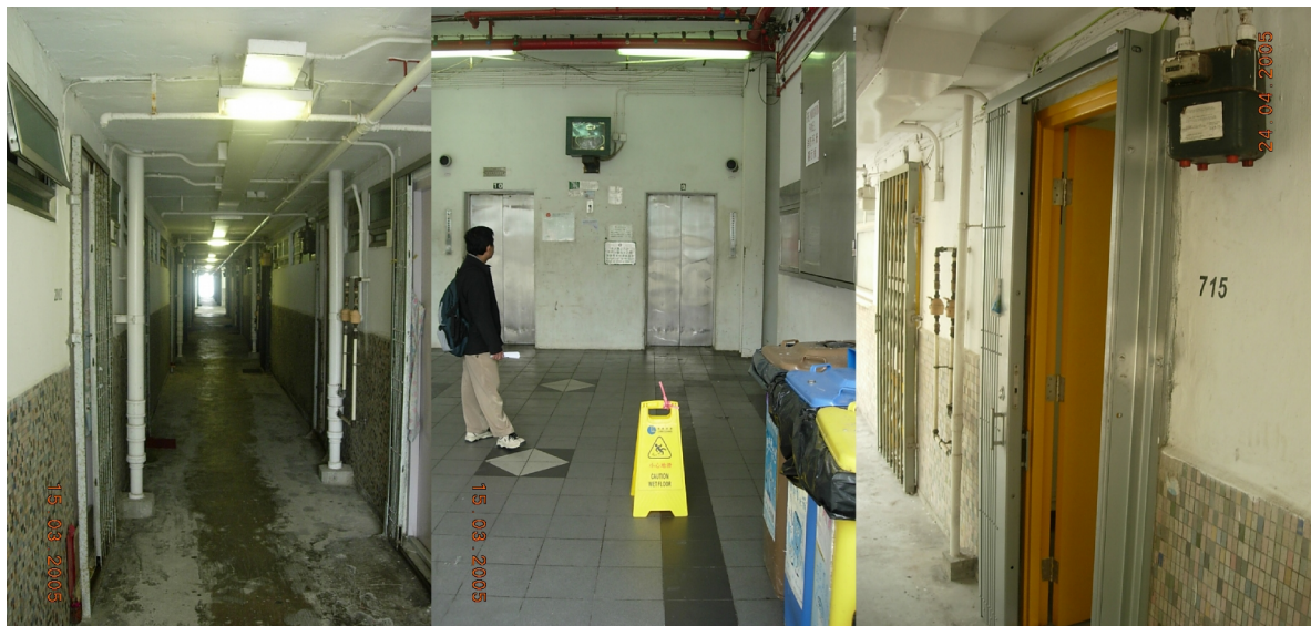
Figure 5. Circulation spaces a) Lift lobby b) dark double loaded corridor, and c) bright single loaded corridor
